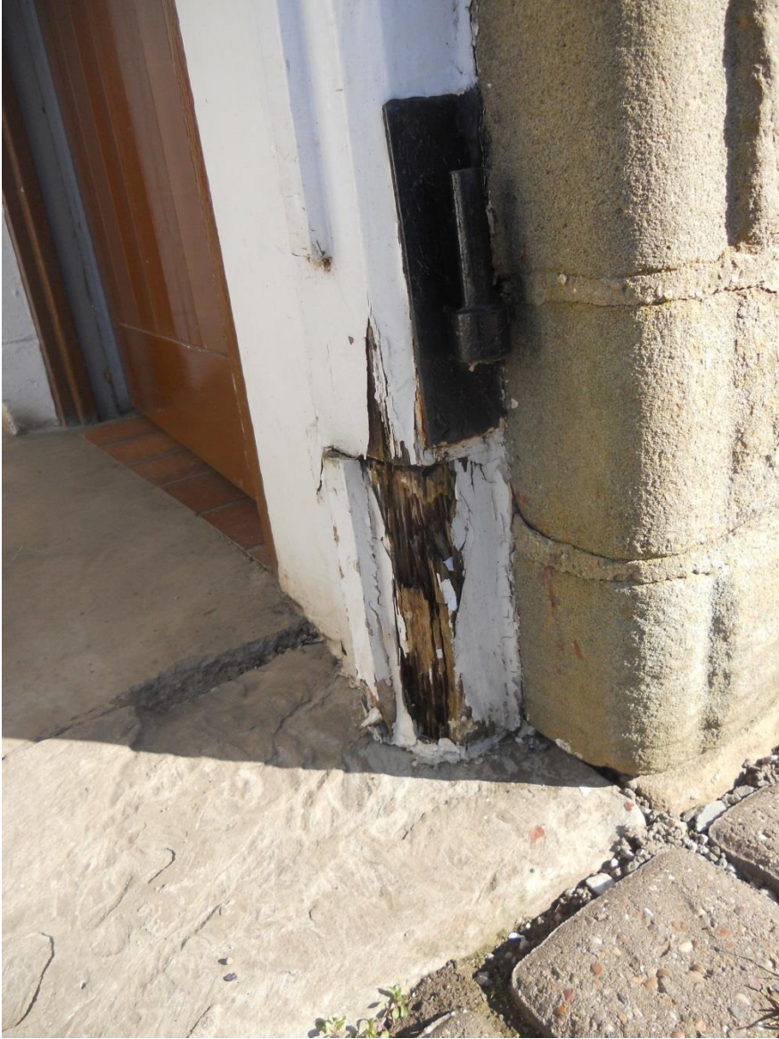
ROT TO DOOR FRAME – BOOKING OFFICE
